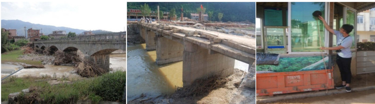
Figure 5. The river way of Macuo Village (left), the destroyed Bridge of Longfenggu (middle), the service center of Xiaguang drifting company (right).
