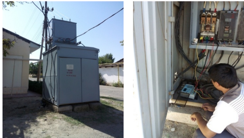
Figure 2. General view of the transformer sub-station where measurements were taken.
