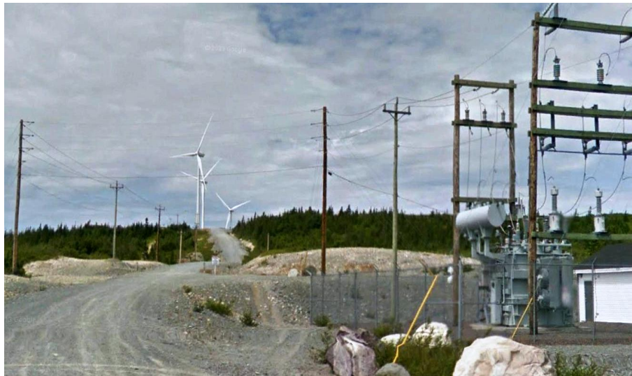
Figure 6. View of the wind farm from its transformation station.
