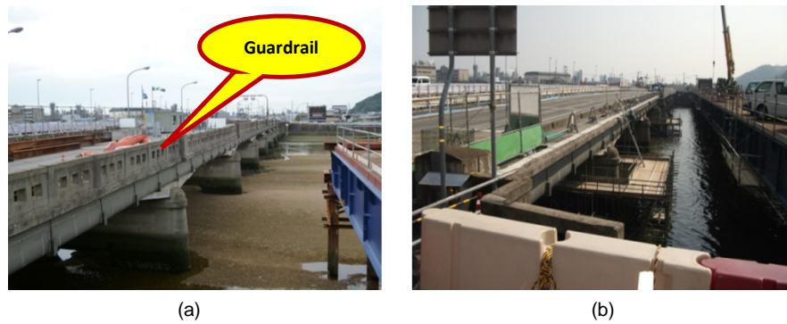
Figure 30. Bridge before and after guardrail removal. (a) Before guardrail removal; (b) After guardrail removal.
