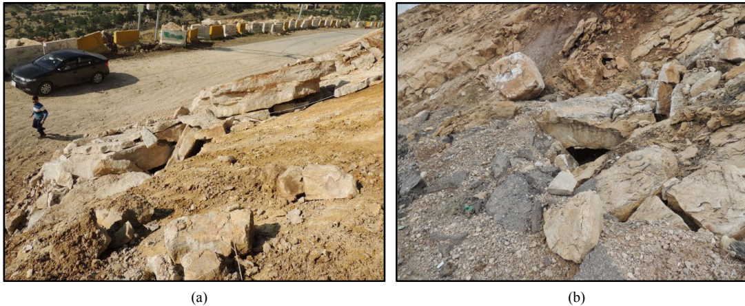
Figure 6. Toe area of Koya Landslide, (a) The remains of the toe area, (b) Blocks of the toe area impregnated in the paved road.
