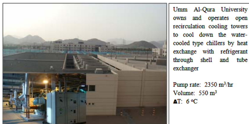
Figure 5. Open recirculation cooling towers at UQU.
