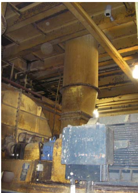
Figure 2. View of the studied equipment. The casing of the blower is visible far left; the two main bearings are visible left (one black, one blue); the motor is at the right; above is the casing of the thermographic camera.
