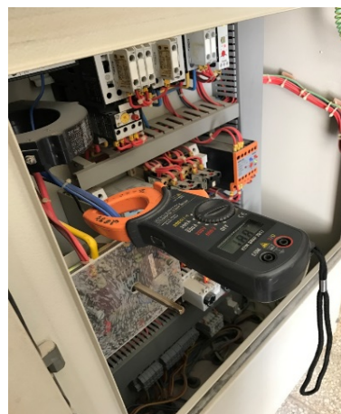
Figure 6. Clamp meter used to measure the voltage and current (the photo is taken by authors).
