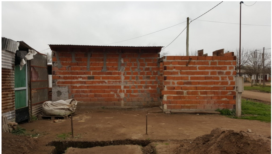
Photo 9. Barrios Unidos: rehabilitation of a house in a social housing development (Source: Photo Teo Vexina Wilkinson, CODEV, 2017).
