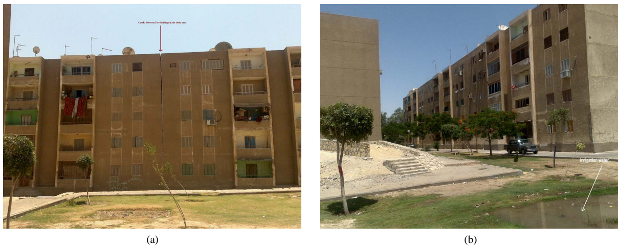
Figure 16. (a) Crack between two sides of building in the study area; (b) The water pool used in the irrigation of garden between buildings in the study area.
