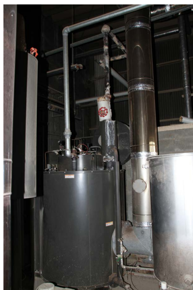
Figure 7. Technically advance boiler used for steam generation.
