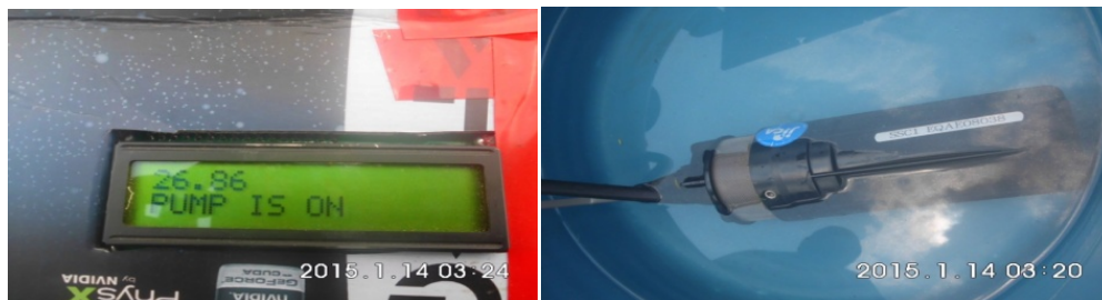
Figure 4. Pump is ON while rising water from low level to high level in the storage tank.
