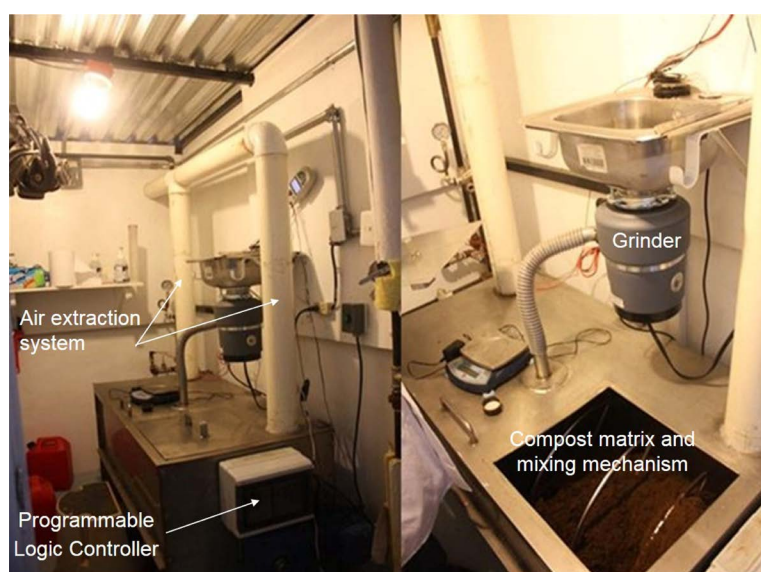
Figure 1. Pilot of a thermal aerobic treatment system installed at the San José hospital. Monterrey, Mexico.
