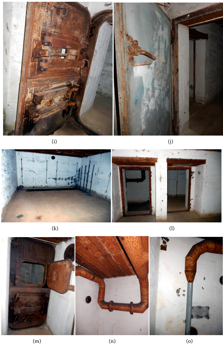
Figure 4. L410A (a) vision from the 1 st VZa ; (b) access stair to the entrances; (c) entrances with circular, armored air intakes and rectangular slabs covering the drainage system, on the left metallic coverage of the close combat room; (d) metallic coverage of the close combat room, details; (e) L410A plan: 1. gasloch, 2. close combat room, 3. crew room, 4. ammunition room, 10. Flak gun emplacement, 22. ventilation room, 33. non-commissioned officer room (Rudi, 1998); (f) gun embrasure of the close combat room; (g) drainage system at the interior; (h) gas loch entrance armored door; (i) other gas loch entrance armored door; (j) other gas loch exit armored door, crew room and single communication door between the crew rooms; (k) crew room, on the upper side of the wall hole for a Festungssofen WT80 conduit; (l) on the left ventilation room, on the right non-commissioned officer room; (m) armored door of the close combat room; (n)-(o) ventilation room with portions of the original ventilation system conduits.
