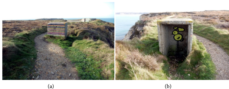
Figure 14. Latrine (a) rear side with R636a in the foreground; (b) front side.
