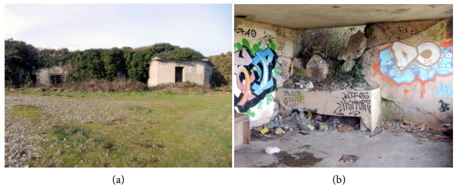
Figure 19. Three concrete barracks, probably of French construction (a) entrances of the west and east barrack; (b) east barrack interior, possible canteen.
