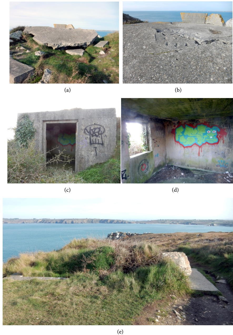
Figure 8. Grand Gouin pointe (a) platform, collapsed portion; (b) platform, fracture line and incisions; (c) barrack near the platform; (d) interior single room; (e) rectangular component of unknown purpose, on the left the Goulet mound, in the middle the Grand Gouin pointe.
