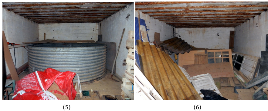
Figure 13. M134 (21)-(1) entrance with concrete access ramp and protection walls, (2) M134 plan: 4 ammunition room (Rudi 1988), (3) corridor with ammunition room entrances and metallic ceiling, (4) room door, (5) ammunition room, (6) ammunition room.
