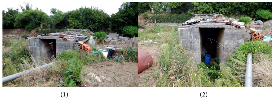
Figure 14. Vf (22)-(1) entrance with access ramp without protection walls, (2) entrance obstructed by vegetation.
