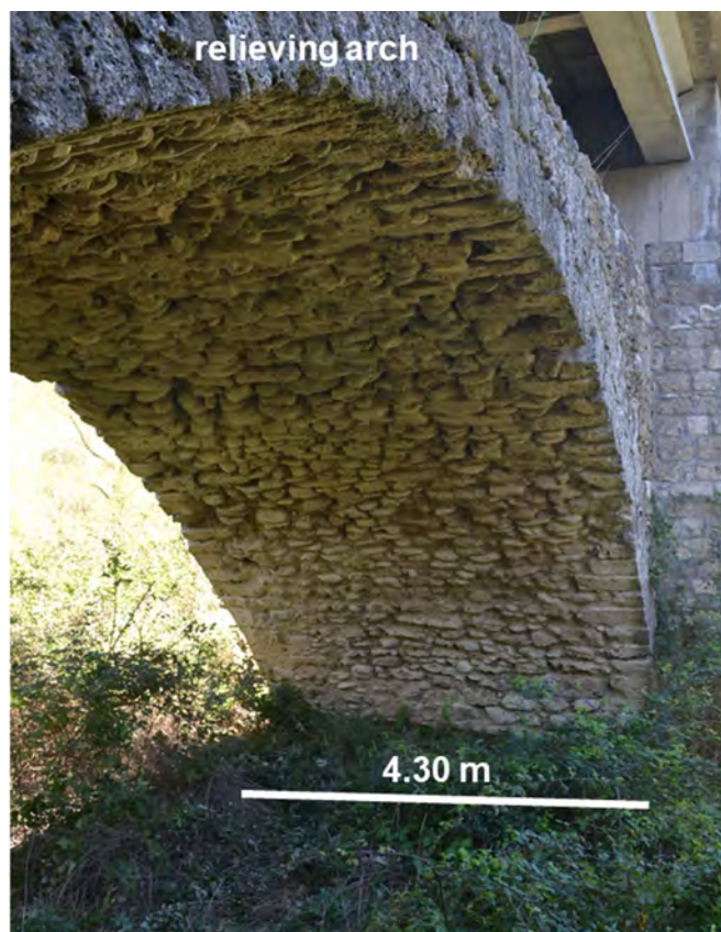
Figure 8. Face of the arch 3, 4.30 m wide, showing the opus incertum , consisting of marly and siliceous limestone pebbles with a blade shape and tiled structure, and the relieving arch with the squared ashlar of phytoclastic travertine.
