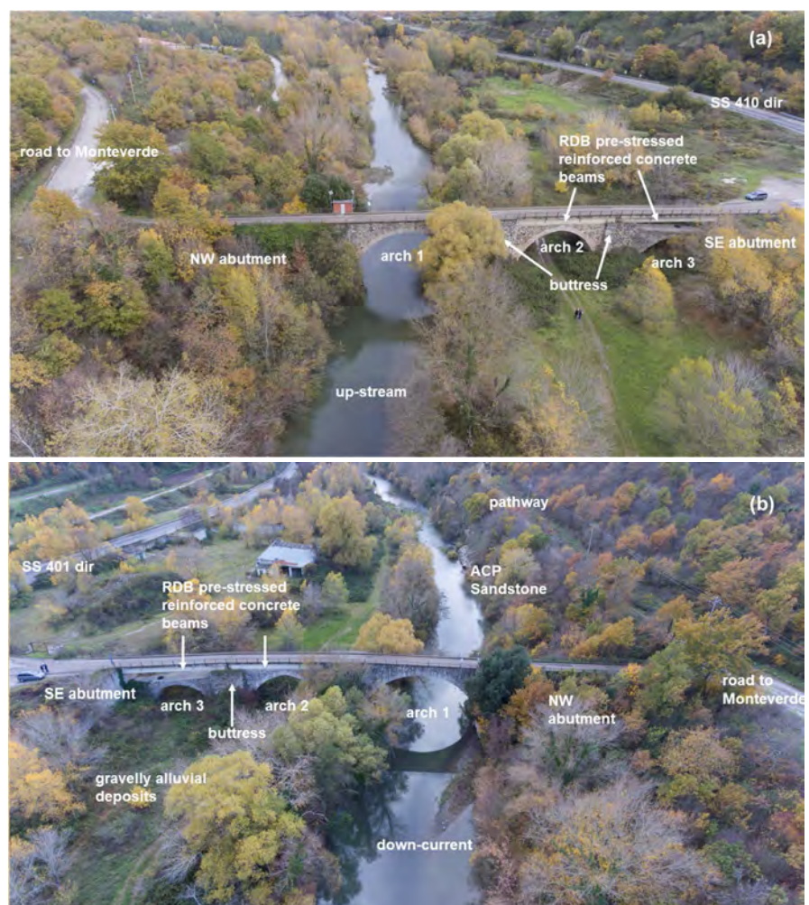
Figure 6. Current state of the façade of the POB as seen through the drone up-stream (southwest) in (a) and down-stream (northeast) in (b). The abutments, the arches 2 and 3 and the cutwaters are covered by weed and climbing vegetation. The pathway in (b) coincides with the layout of the old Appian Way.
