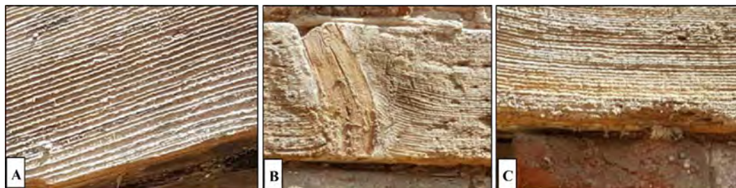
Figure 9. The lintel of the door in the mausoleum dome chamber (A) The roughness of weathered wood surface, (B) the wood knots affected by weathering, (C) the spongy appearance of the wood surface and the erosion of lintel edges.
