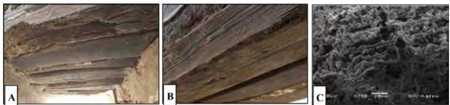
Figure 2. (A)-(C), shows the burn of some window lintels in the outer portico of Fatma Khatun mausoleum, (C) SEM micrograph. 20 \mu\text{m} .
