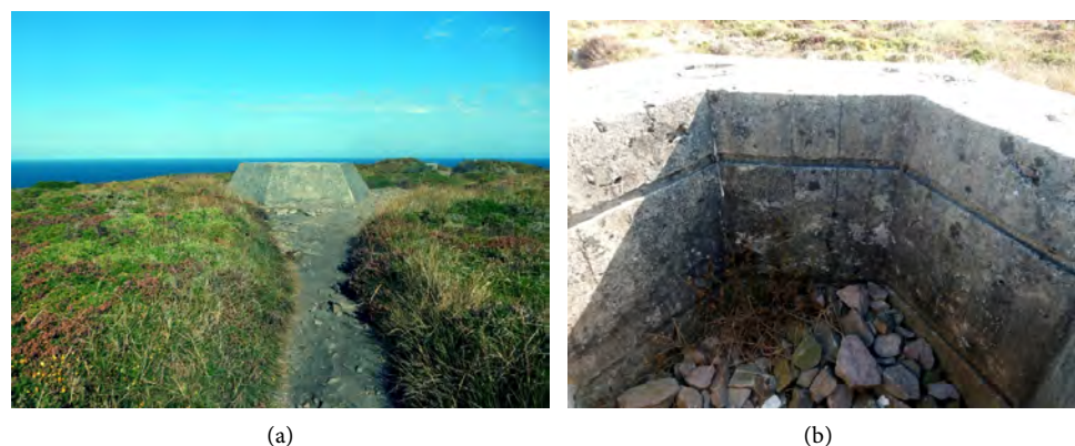
Figure 5. V 229 (4): (a) support for Würzburg Riese ; (b) interior walls with two recesses for shelves or equipment.
