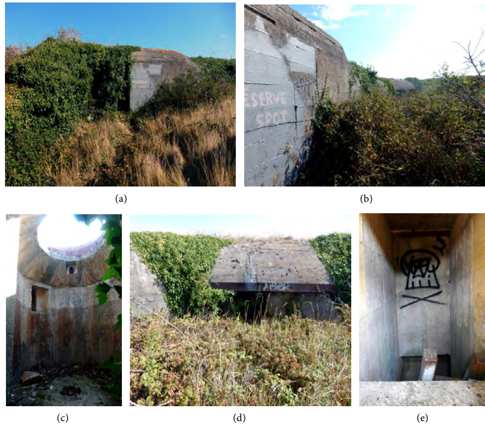
Figure 8. L 479 bunker (10): (a) observation post entrance; (b) façade; (c) observation post interior; (d) façade detail; (e) re-cooling room conduit with original white painting.
