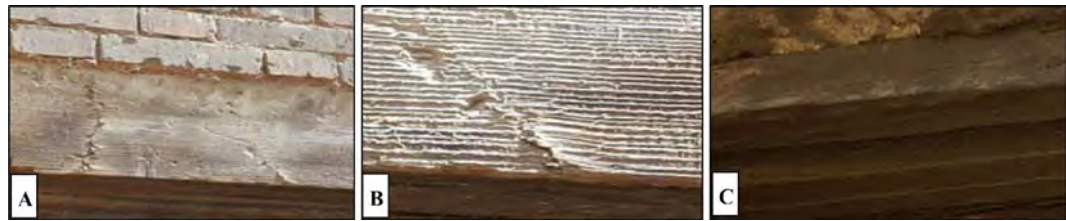
Figure 6. Spread of the different cracks on the pine wood surface, ((A), (B)) the lintel of the door in the mausoleum dome chamber, (C) the window lintel in the outer portico.
