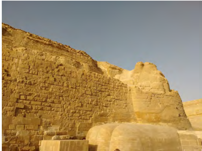
Figure 13. The repaired (beginning with Baraize, circa 1926) major fissure through the left waist of the Sphinx as seen from the north. Photo by M.S., June 2019.
