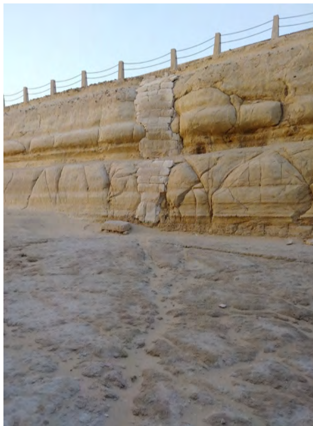
Figure 12. The southern extent of the major fissure through the enclosure wall viewed from the northwest along its course through the ditch floor. Modern masonry repairs have covered the fissure. Photo by M.S., June 2019.
