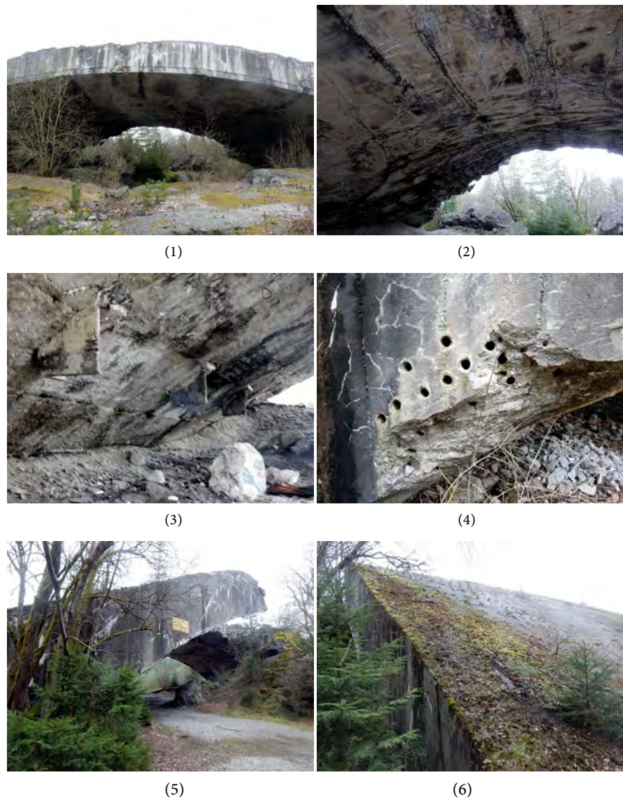
Figure 6. Weingut I—7 th arch: (1) coverage rear side with 30 cm and 5 m concrete layers, in the foreground 6 th arch coverage; (2) coverage with constructive segments; (3) coverage with constructive segments and aligned vertical protrusions; (4) dynamite holes on the rear side; (5) rear side with empty space of the fallen part and attached part; (6) coverage with aligned armour iron extremities.
