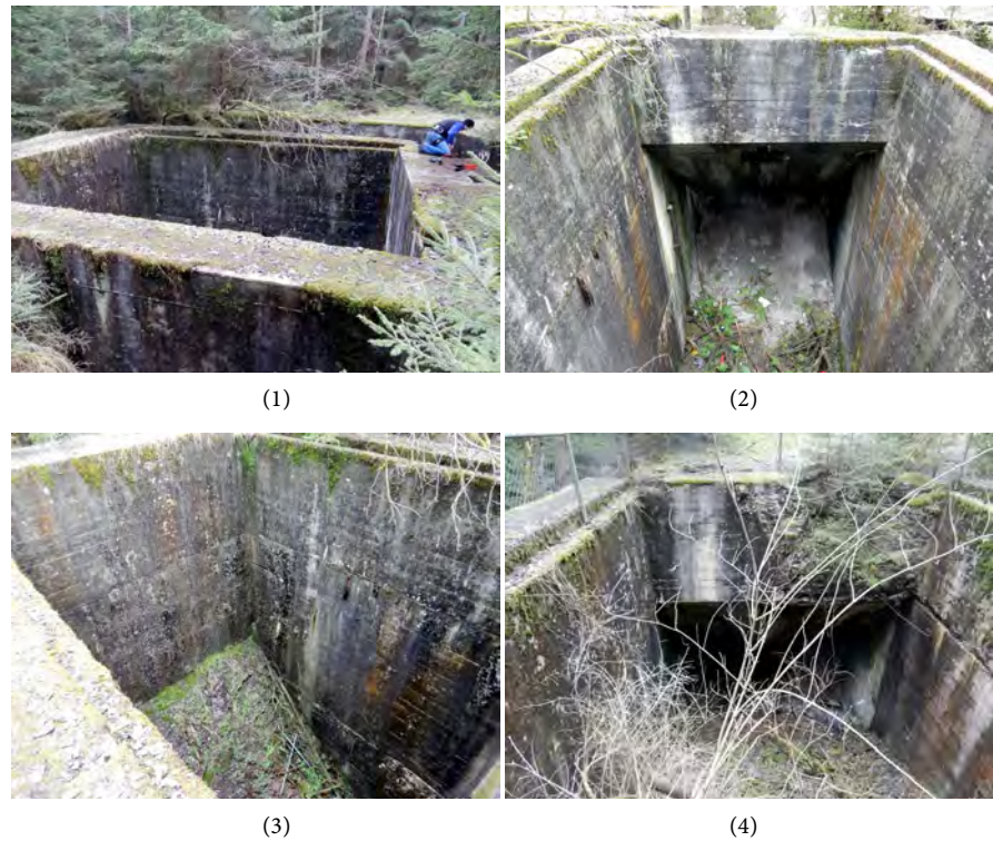
Figure 9. Weingut I —(1) first air intake/exhaust, square internal wall; (2) well entrance toward Weingut I ; (3) well inclined floor; (4) second air intake/exhaust.
