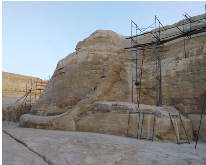
Figure 11. The repaired major fissure on the south side of the Great Sphinx's waist can be seen to course through the hind paw and on through the ditch. Photo by M.S., June 2019.
