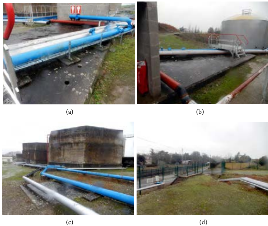
Figure 17. Bouchemaine oil terminal—(a) bunker i crossed by pipes, west view; (b) bunker i crossed by pipes, east view; (c) possible buried bunker under pipes; (d) pipes exit toward the freight station, in the foreground left the Bouchemaine passenger station.
