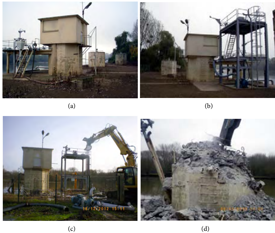
Figure 9. Pumping station and bollard c demolition—(a) side view, on the left the added metallic platform with oil discharging tubes, on the foreground right the columnar bollards d, e (courtesy Mr F. Guillaume, 07 th November 2006); (b) side view, on the foreground left the columnar bollard b, on the right the metallic platform with oil discharging tubes (courtesy Mr F. Guillaume, 07 th November 2006); (c) platform and pumping station demolition (courtesy Mr F. Guillaume); (d) bollard c demolition (courtesy Mr F. Guillaume).
