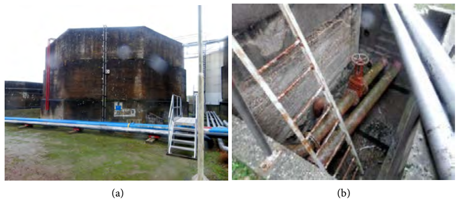
Figure 14. octagonal wall D—(a) external structure with white board covered by a square, blue board; (b) concrete pit with connection pipes.
