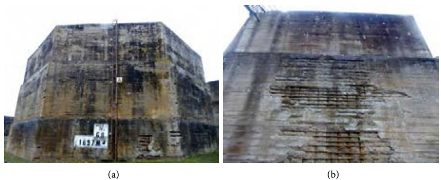
Figure 13. Octagonal wall A—(a) three steps external structure with white board; (b) local concrete superficial failures.
